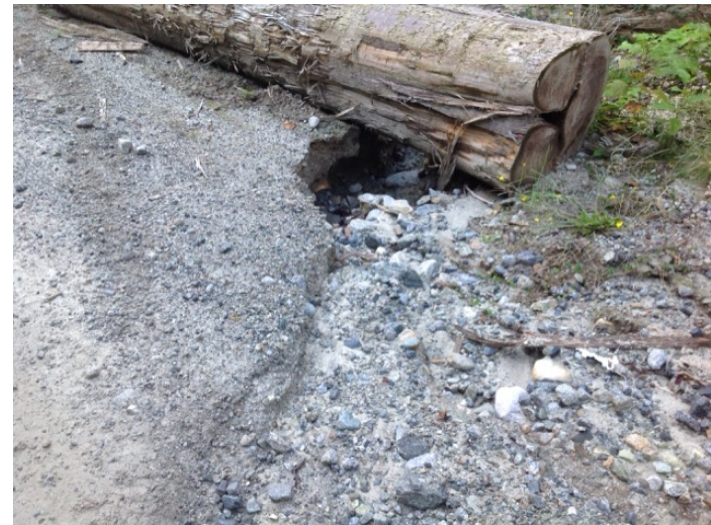
right approach down stream erosion
