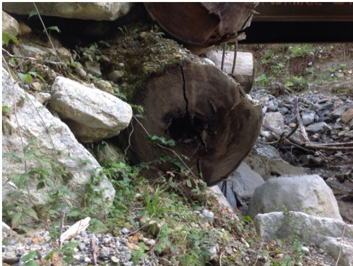
right bank abutment, 3rd crib log crack
